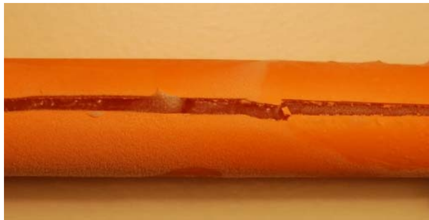
Figure 7. Picture of frozen CPVC pipe.
