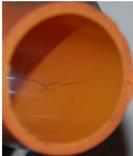
Figure 1. Formation of a stress-crack on the inside of a CPVC fire sprinkler pipe at a point where a tight-fitting clamp was used.
