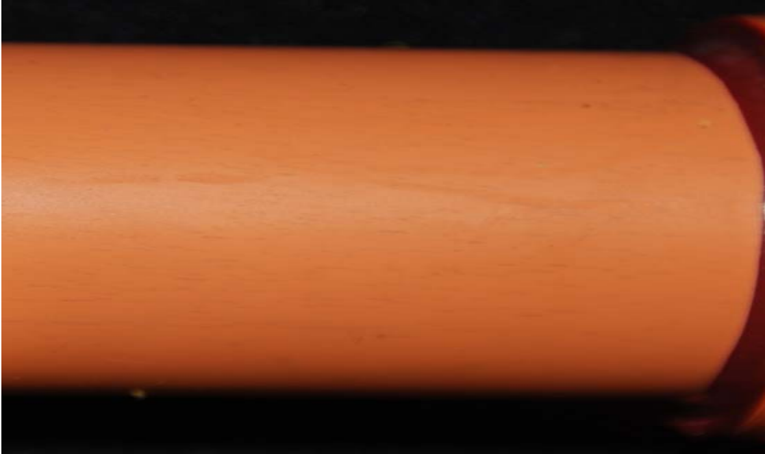
Figure 17. Extensive surface crazing of outside pipe wall.
